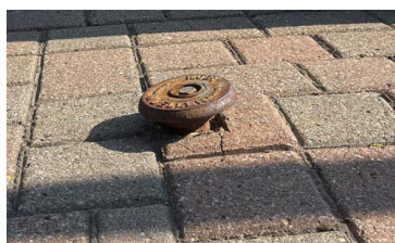
Potential trip hazards for pedestrians.
